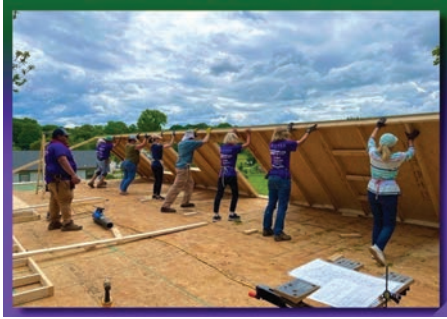
Governors Club volunteers and others help raise the roof for Chatham Habitat.
